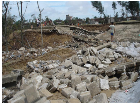
Hoang Hoa dike (Thanh Hoa) after typhoon 7/2005
