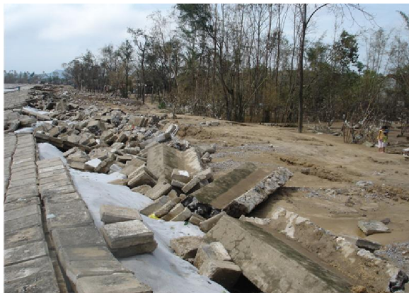
Hau Loc dike (Thanh Hoa) after typhoon 7/2005
