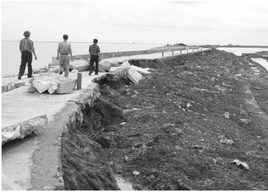
Wave overtopping caused inner slope erosion in typhoon no. 7/2005 at Cat Hai (Hai Phong)
