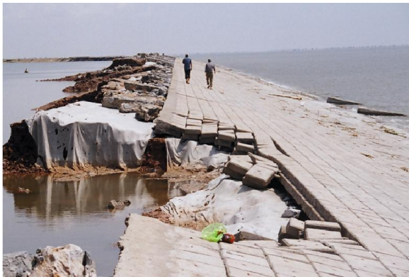
Co Vay (Nam Định) dike after typhoon 7/2005
