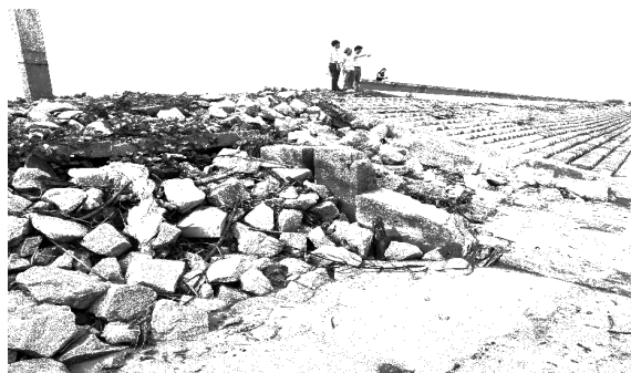
Figure 4: Failed dyke profile location B (Source: Own archive, 2017)
