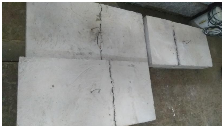
Fig. 9. Flexural failure in unreinforced and TRC-strengthened reinforced concrete slabs.
