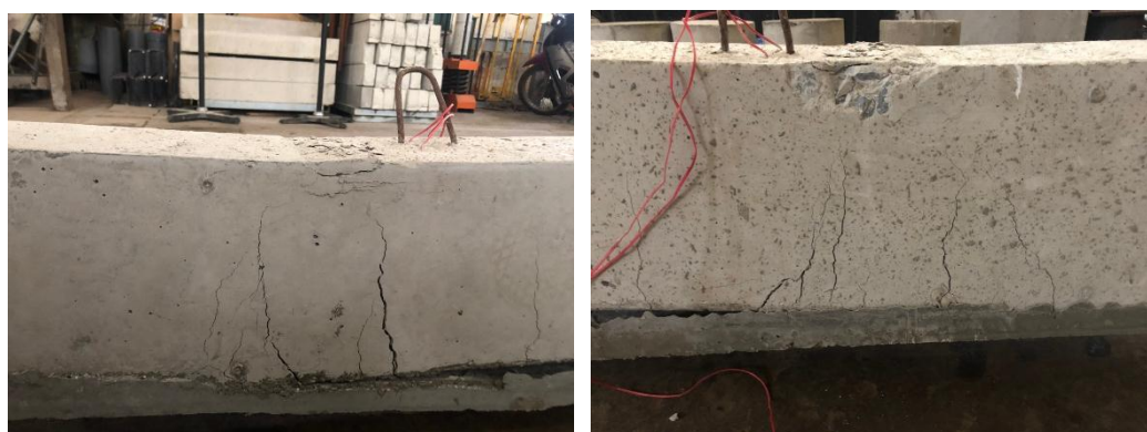
Fig. 11. Flexural cracks in the strengthened beam and failure of the compressive concrete in the strengthened beam.
