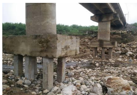
b) Erosion of bridge pier foundation in Ky Anh - Ha Tinh
