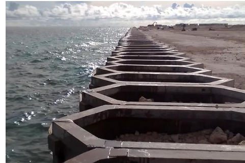
Fig. 6. The tank is moved to the construction location by crane after completion of installation.
