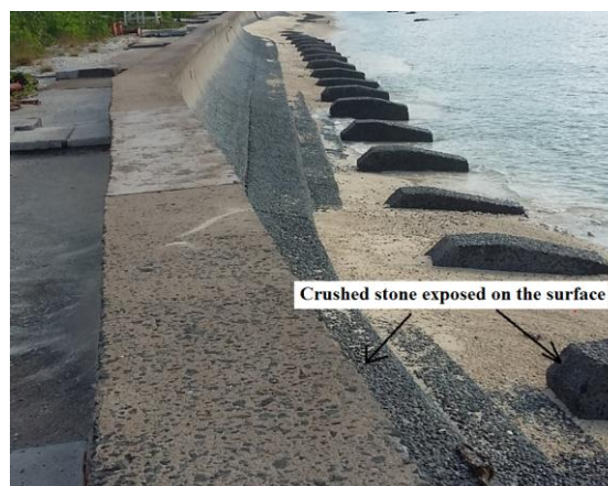
Fig. 1. Gravity revetment made of concrete poured in place on an offshore island in Vietnam after more than 30 years of exploitation.
