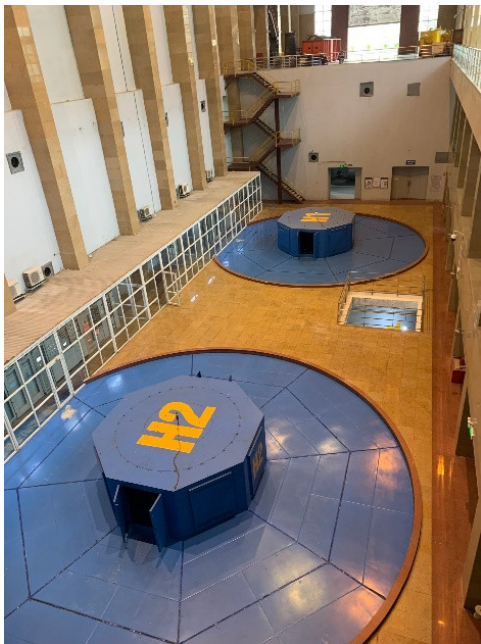
Fig. 8. BanVe hydro turbine units - H1,H2
