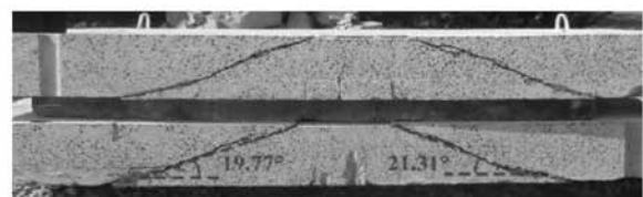
Fig. 21. Depicts patterns of failure for LD and LA slabs as shown in the experimental and FE models.
