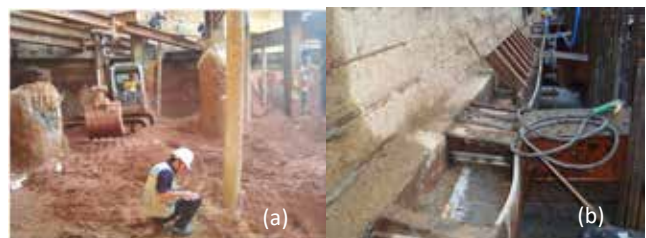
Figure 7. (a) under excavation of B3; (b) The 3 rd level of waling beam & struts status
