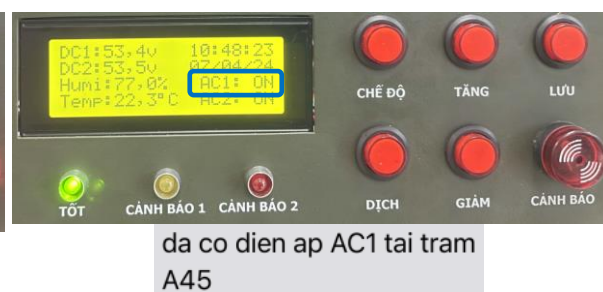
Figure 12. Respond of device when AC power is restore
